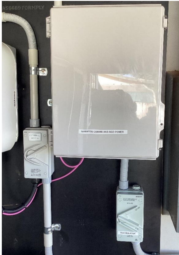
Figure 5: Example SGD installation
